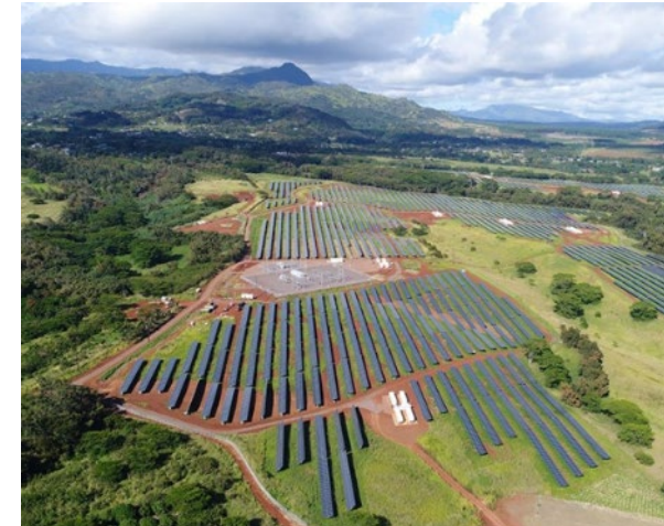
PV-Storage Microgrid, 28 MW, Hawaii Source: AES Hawai'i
